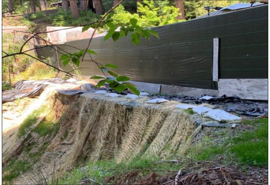
Investigators discovered a landslide below an unpermitted cannabis operation in Boulder
